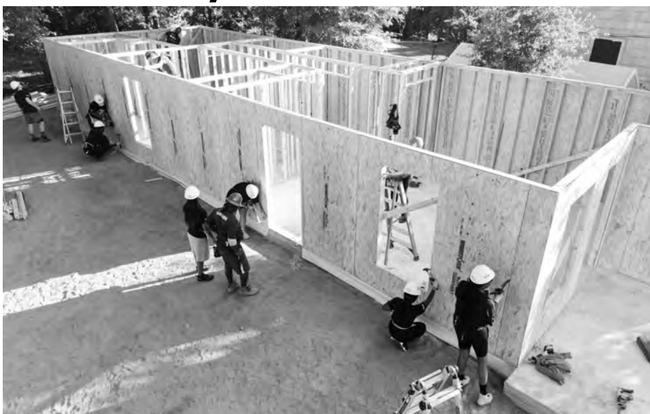
Habitat for Humanity volunteers work together on a Habitat for Humanity home without a roof. Photo submitted
